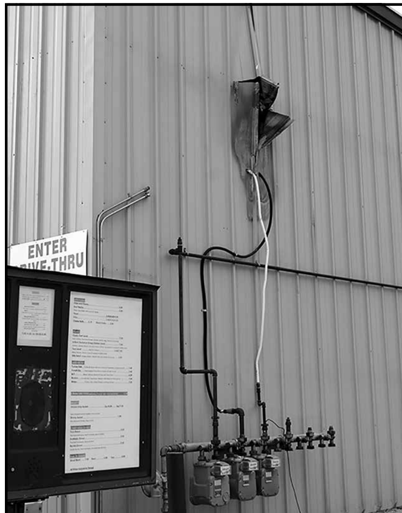
The exterior of the Taco's & More building received damage in a weather-related fire last week.
